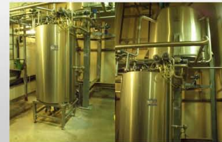
REF M0236 FILTRIX CIP SET WITH 2X TANKS, SHELL & TUBE HEATER, HILGE PUMP, PIPEWORK & VALVES
