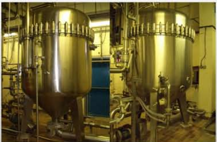
REF FT0243 2 X COMPLETE S/S STELLA-META FILTER STREAMS, 45HL BUFFER TANK, 10HL MIX TANK, PUMPS
